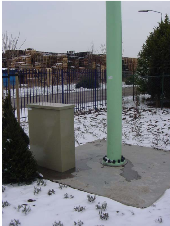
Control Cabinet on Foundation
