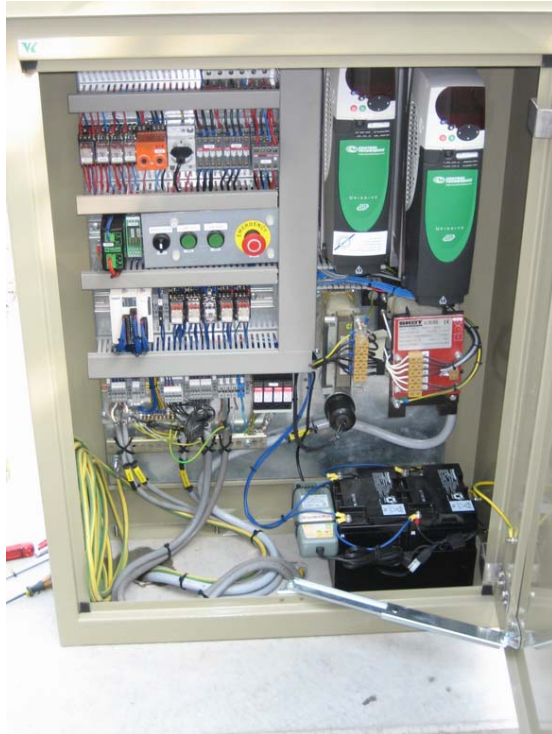
Fully Equipped Control Panel with IGBT inverters
